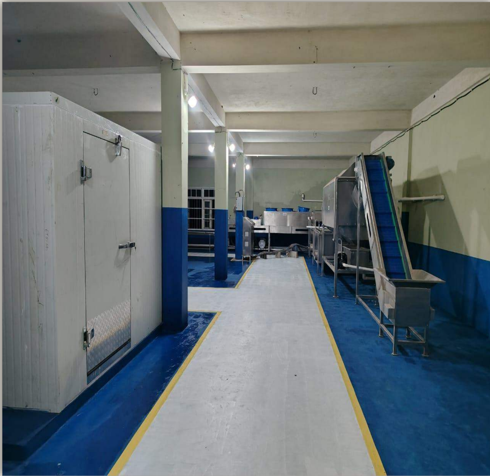
Fig: Processing unit of Ropuiliani WFPCL , MIFCO Complex, Chhingchhip
